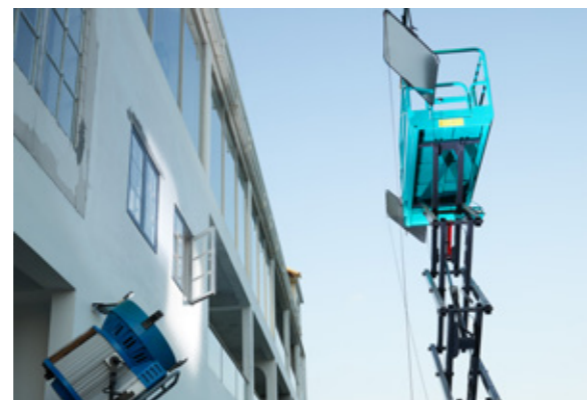
With high-output fixtures in low positions
